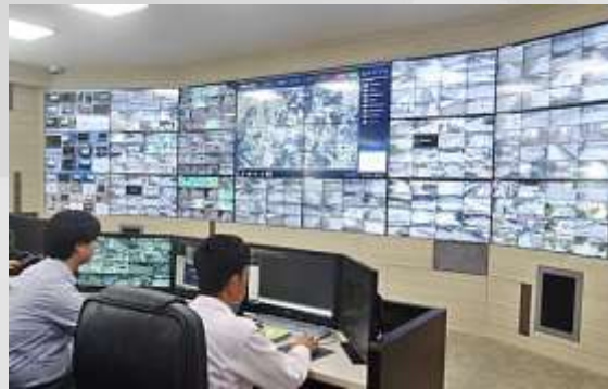
VMS (Video Monitoring System)
